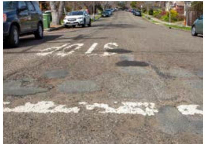
Street Pavement Damage
