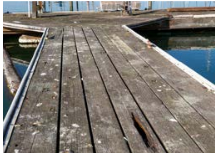
Deteriorated Marina Dock
